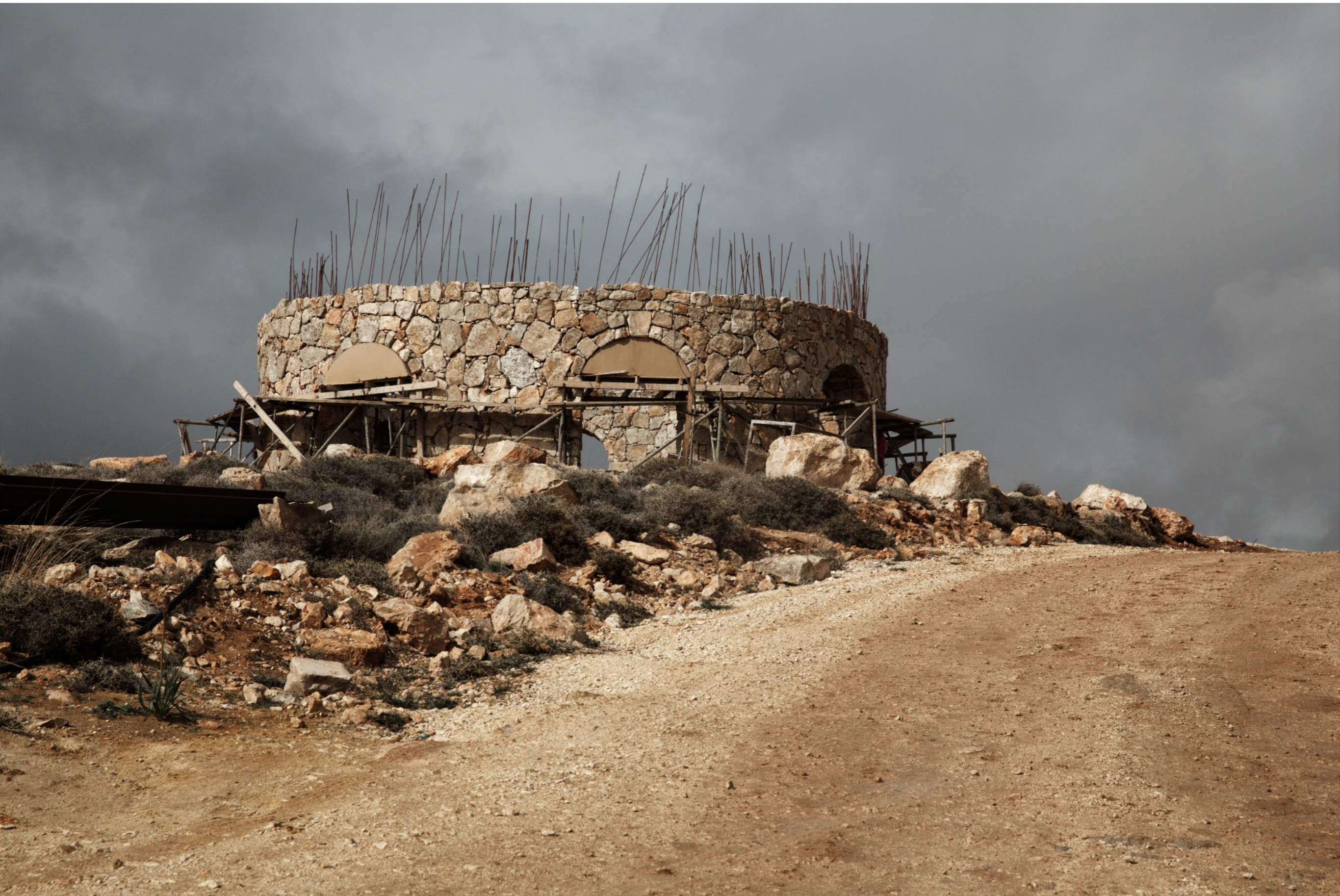
Round-wall synagogue under construction. It is built by Arabs and volunteers from Germany. Arabs are happy that they have this job.
